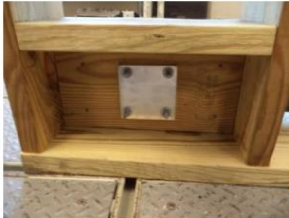
Photo No. 5 Post Mount Installation in Wood Deck - Wood Deck Underside Detail
